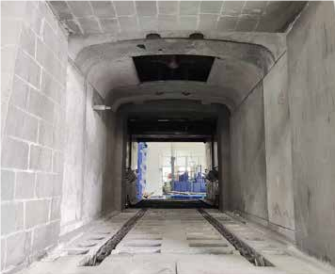
炉膛内部 Furnace Chamber View
